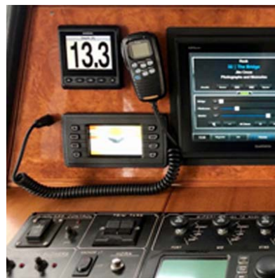
Finished panel where the WESMAR Wave-Smart 3-Axis Gyro is put into action to provide smooth sailing.
