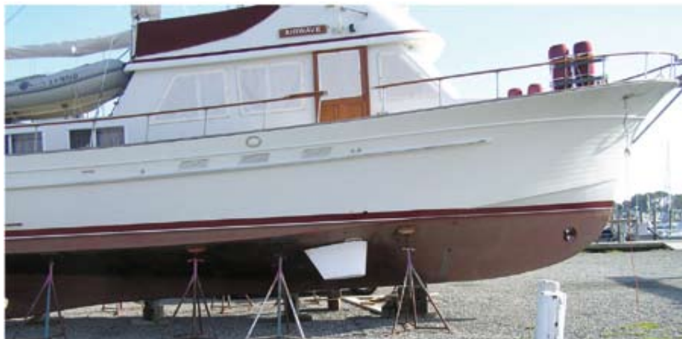
The installation of the WESMAR RS400 Stabilizer System (4.5 ft. square fins) on the MY Airwave went smoothly.
